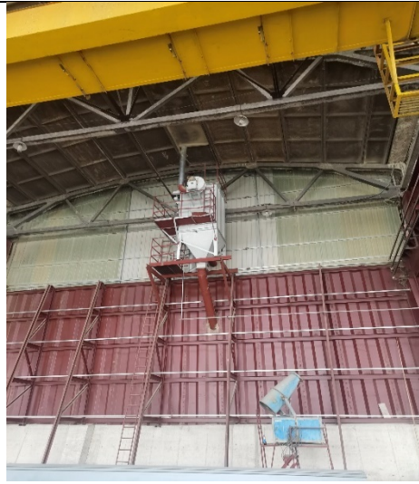
粉煤灰储料仓
